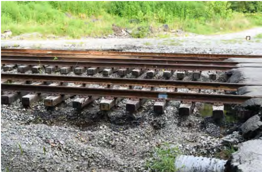
Ballast was washed out in numerous spots. This has been the condition for several years on the inactive segment from Penny, Kentucky, (junction with Damron Fork Mine spur) to Myra, Kentucky.
